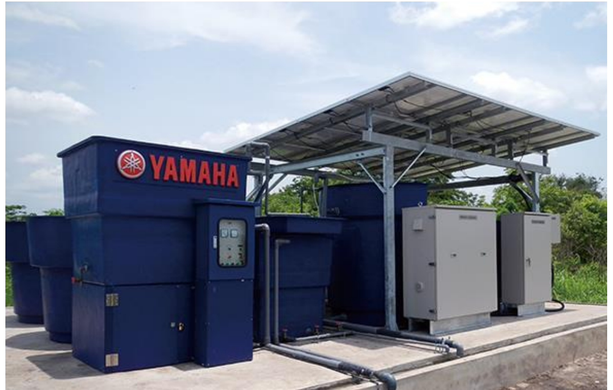
Yamaha Clean Water Supply System
