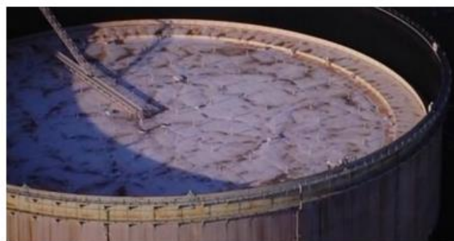
Photo showing the top of a crude-oil reservoir (Source: JXTG Nippon Oil & Energy Corporation)
