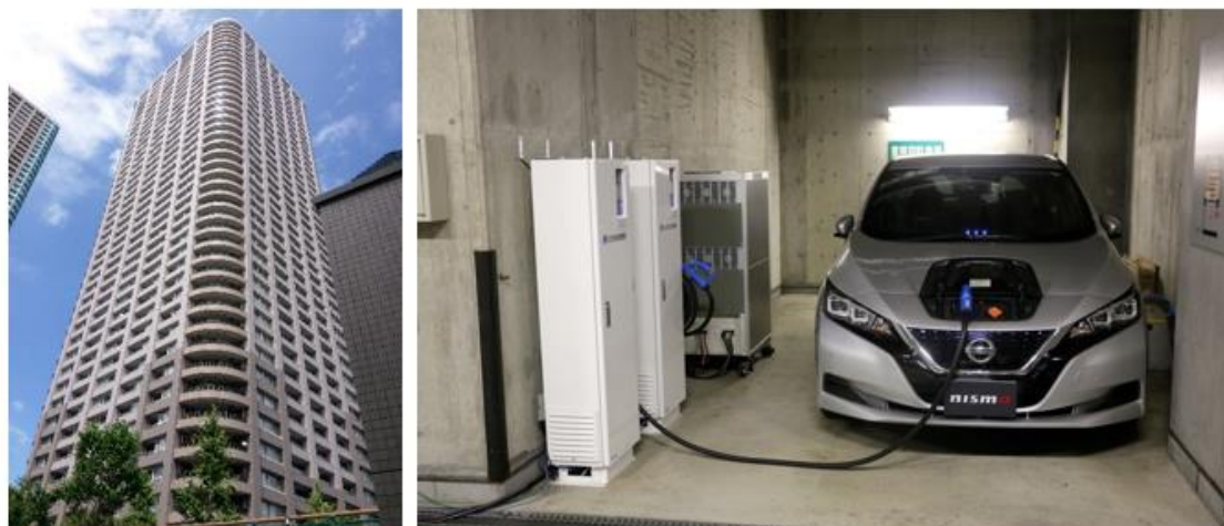
The building and EV2ELV systems used for the experiment
